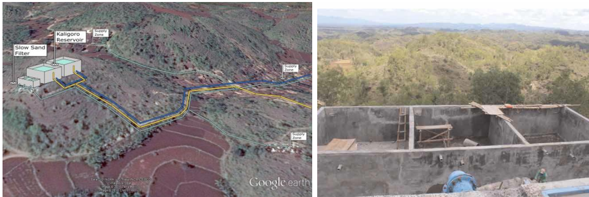
Fig. 3. Location of the slow sand filter beside Kaligoro Reservoir (left), image of the construction phase (right)
